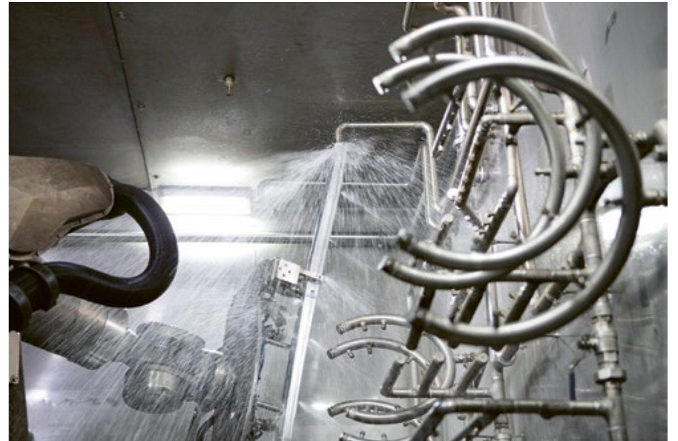
Water sprays from all sides: The robotic arm in the washing cell needs seals that protect its gearbox from extremely fine droplets.
